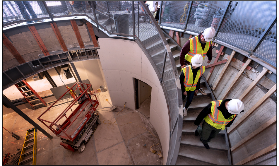
Interior construction is wrapping up on the Mission94 Firearms Education Center. It is expected to open early this summer.
