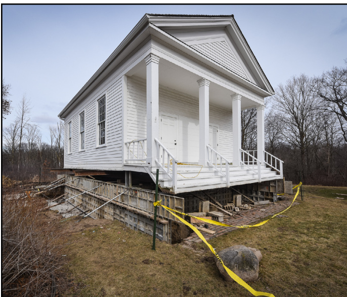
The Somers historic Town Hall is lifted up onto a new foundation. The building is located on the Hawthorn Hollow Nature Sanctuary and Arboretum property.
