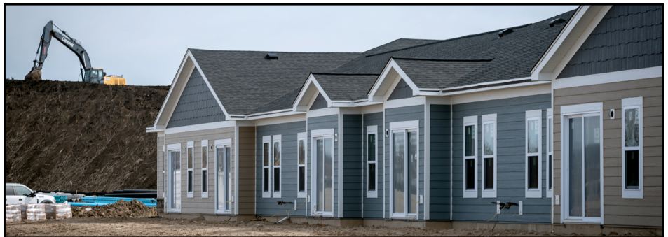
Apartment buildings and a clubhouse are currently under construction at the Savannah at Pike Creek development. It is located at the corner of Green Bay Road and Highway L.
